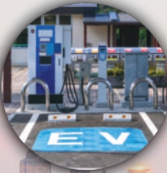
EV Charging Station
